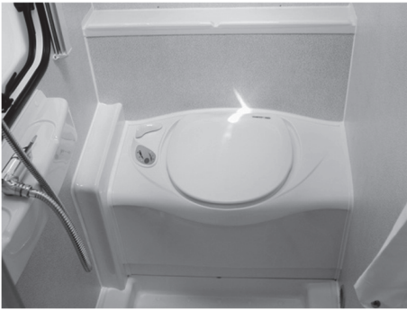
Fig. 48: Toilet, example permanently installed
