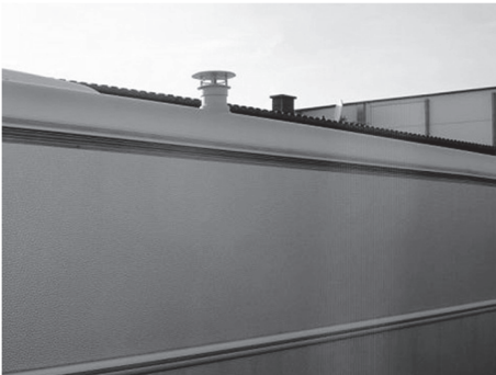
Fig. 84: Exhaust gas stack of the gas heater
