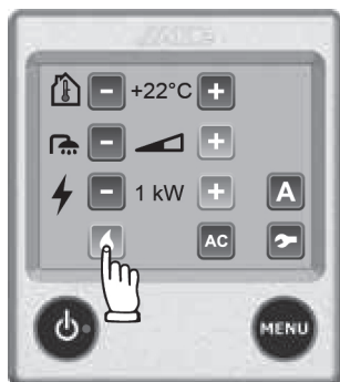
Fig. 169: Heating with gas
