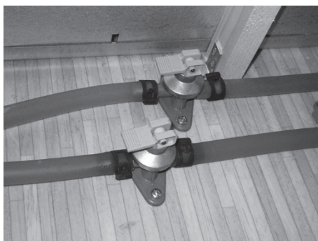
Fig. 178: Closed drain valves
