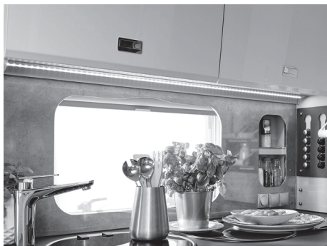
Fig. 67: LED light rail (typical)
